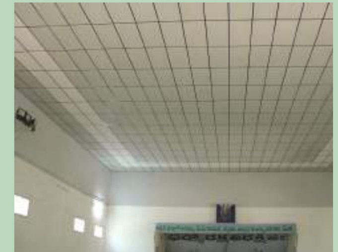
False Ceiling - Grid Type
